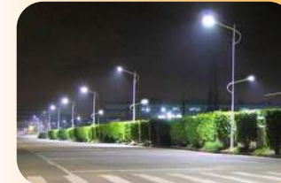
LED Street Lights
